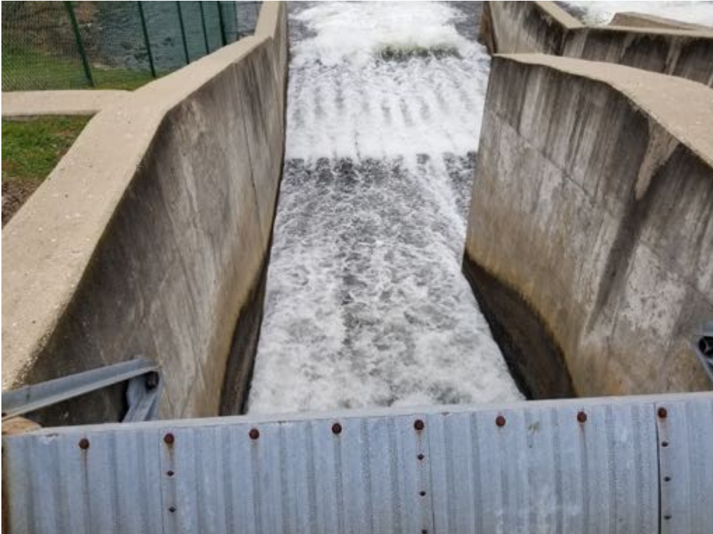
Radial gate looking downstream showing erosion on side walls
