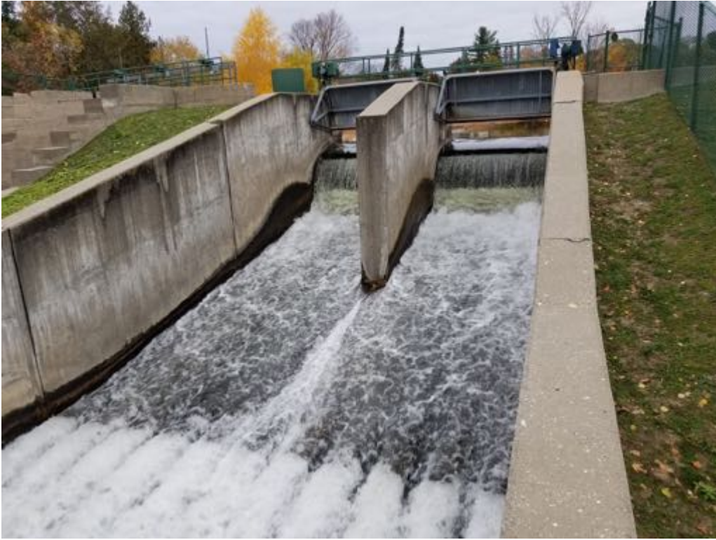
Radial gates looking upstream
