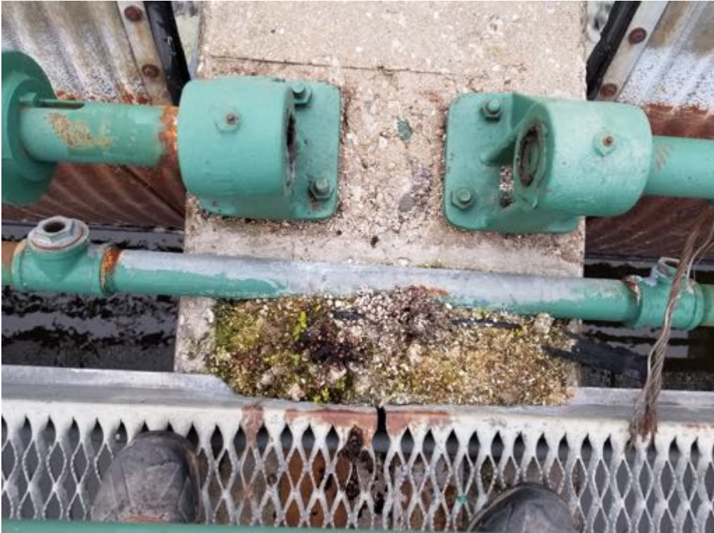
Support section between radial gates showing raccoon feces
