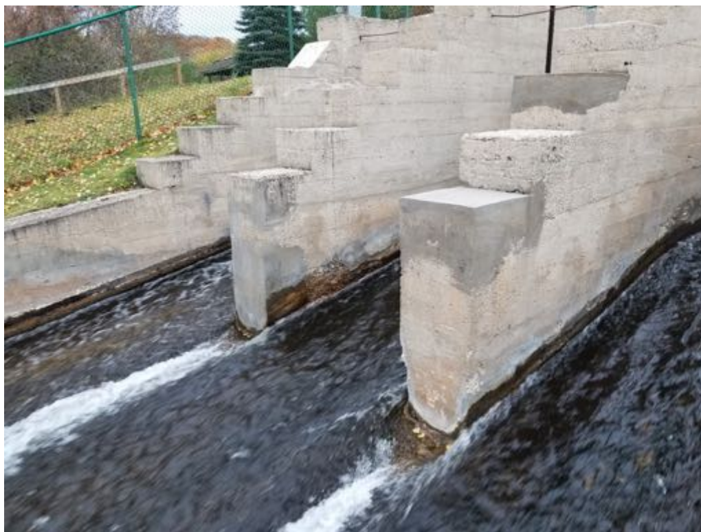
Downstream walls of slide gate discharge sluice showing repairs in good condition
