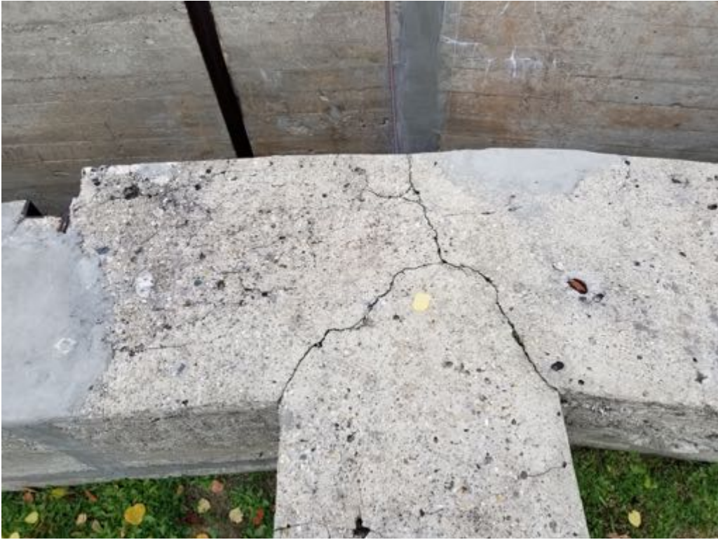
Close up of cracks in concrete that should be repaired and sealed
