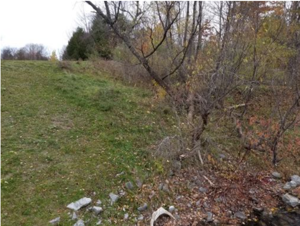
Downstream embankment at east end showing willow trees that should be removed
