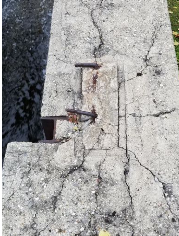
Close up of cracks in concrete that should be repaired and sealed
