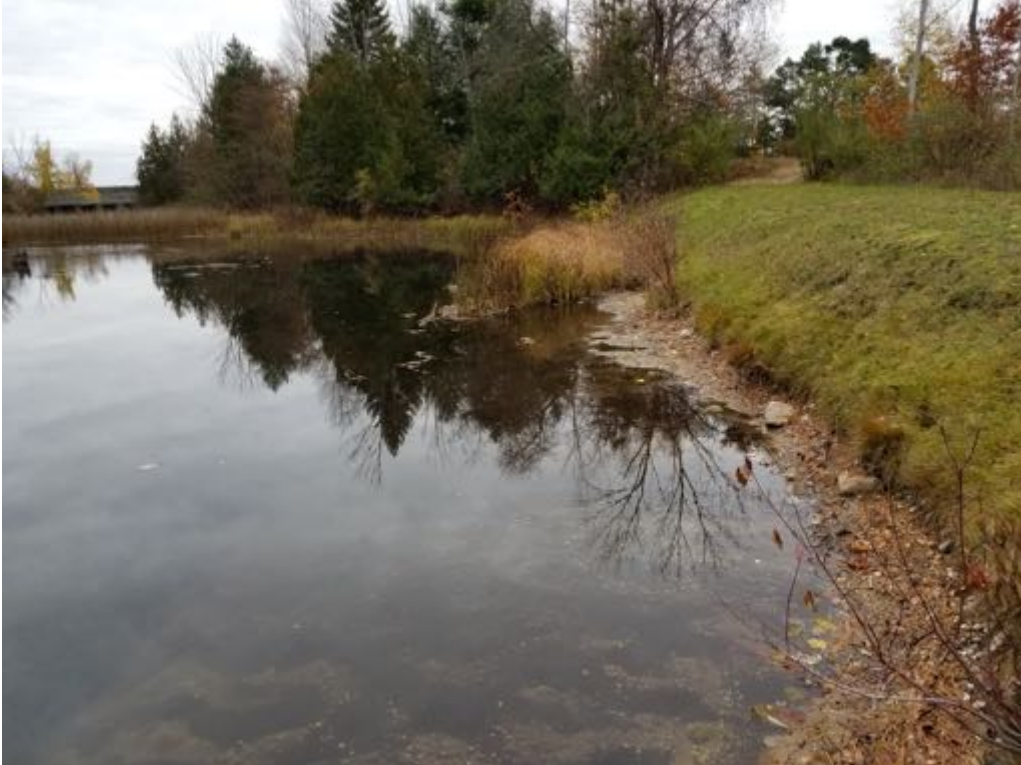
East end of upstream embankment looking east with small willows that should be removed
