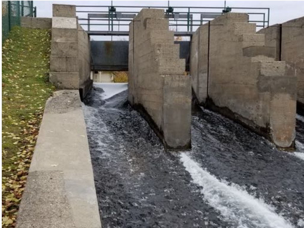
Slide gate discharge chutes
