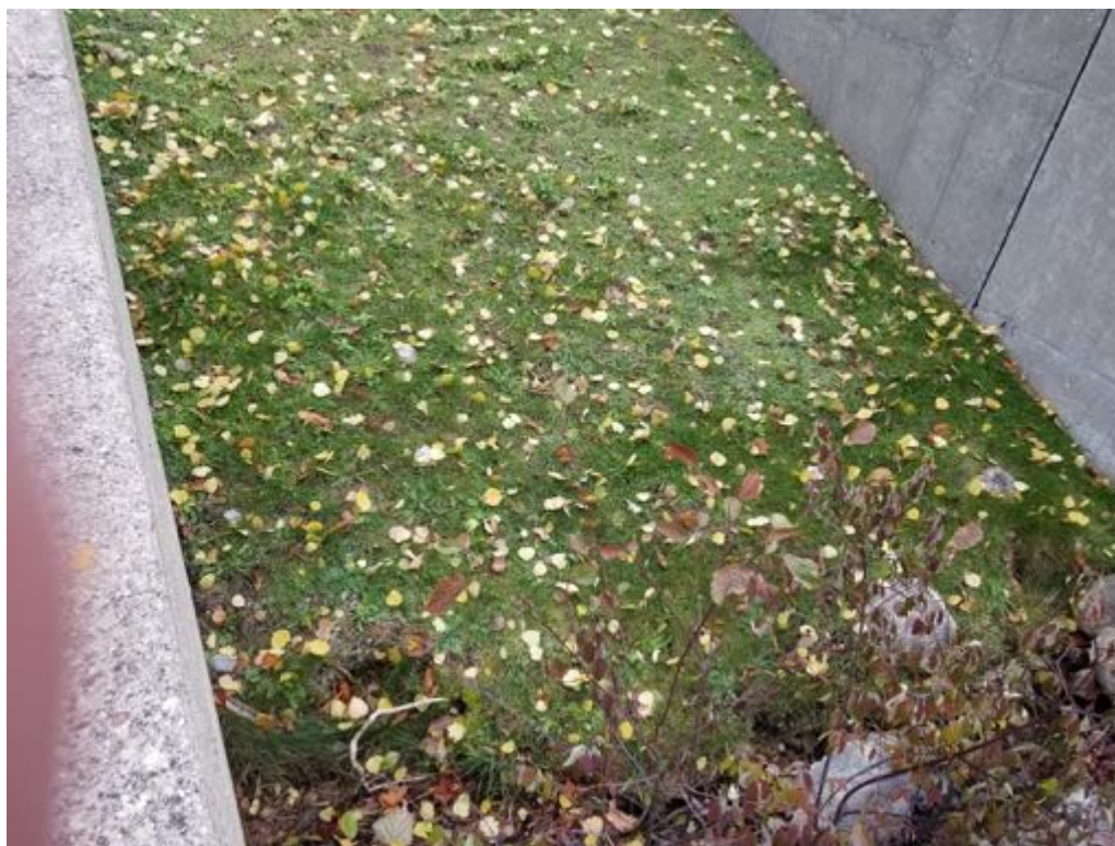
Middle embankment showing woody vegetation that should be removed
