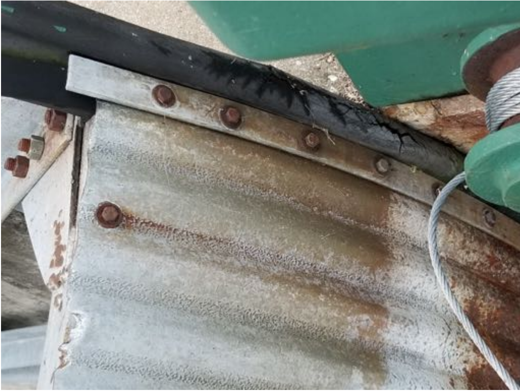
Radial gate showing deteriorated rubber seal along edge of gate
