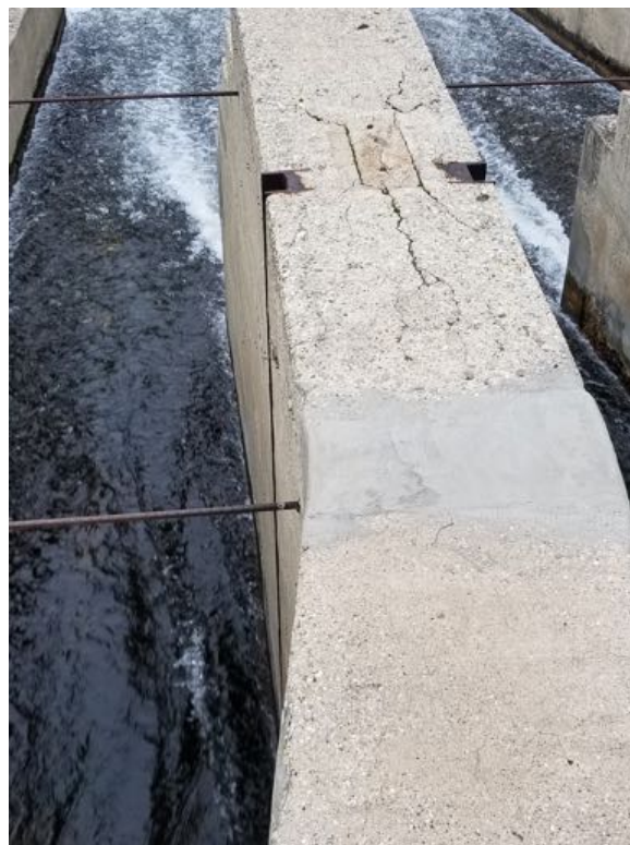
Concrete divider between slide gate discharge sluices showing cracked concrete
